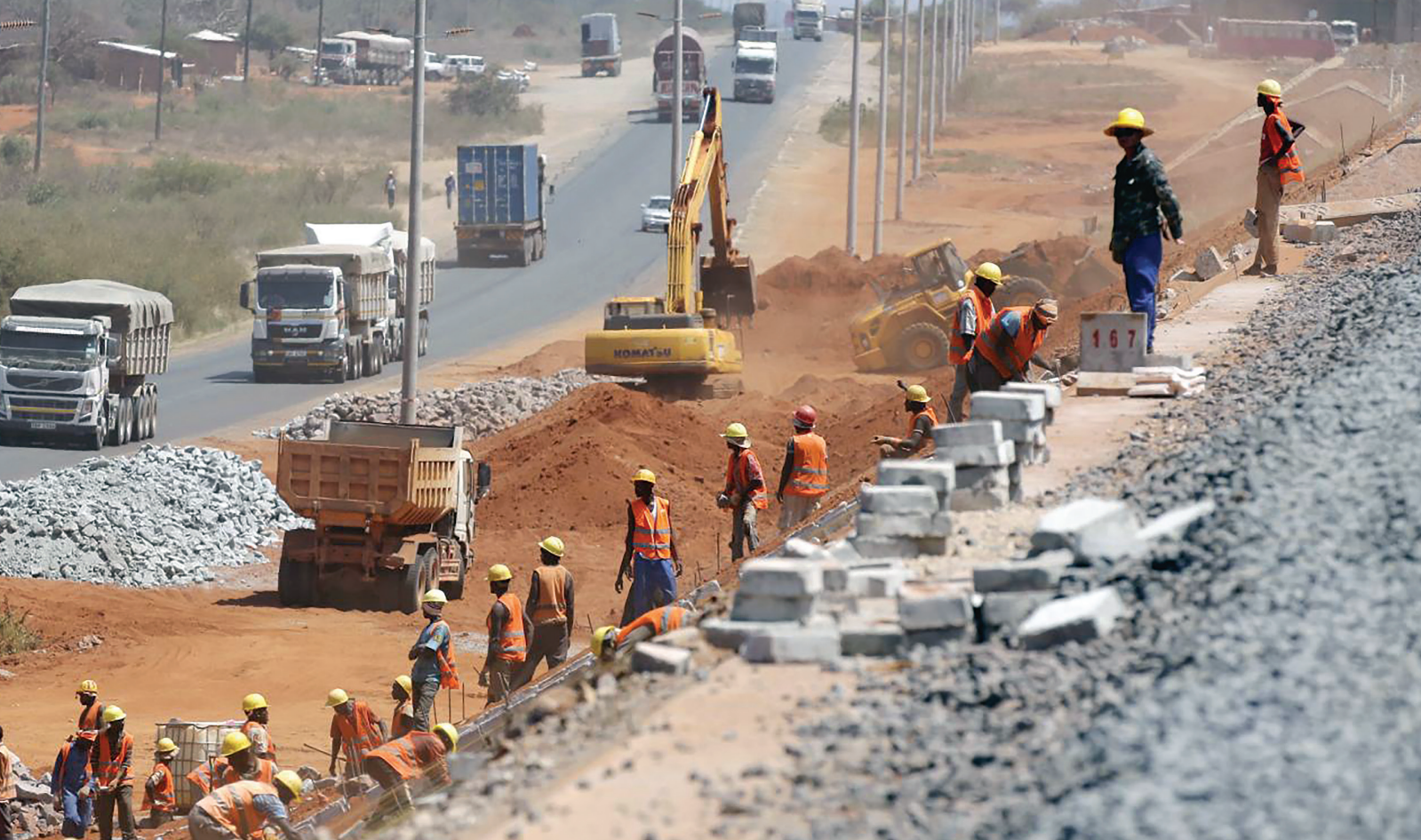
Construction workers work on the new standard gauge railway line near Voi town, Kenya, on March 16, 2016. (Photo Credit: Reuters)
